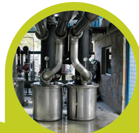
Inside water vapor removal
