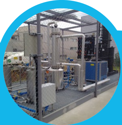
View of energy recovery.
