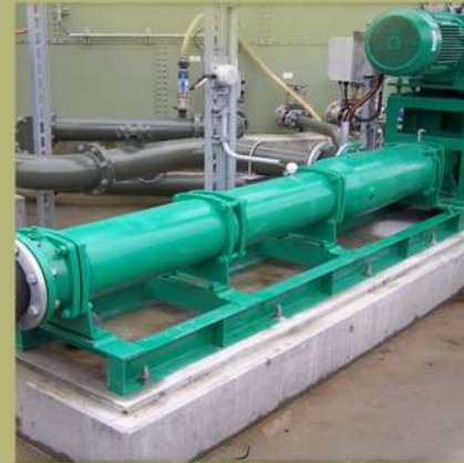
DIGESTATE TRANSFER PUMP
