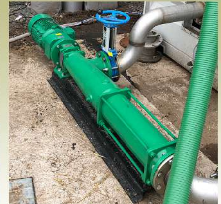
BIOMASS TRANSFER PUMP
