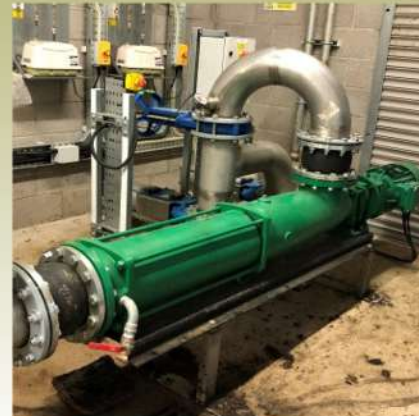
BIOMASS RECIRCULATION PUMP
