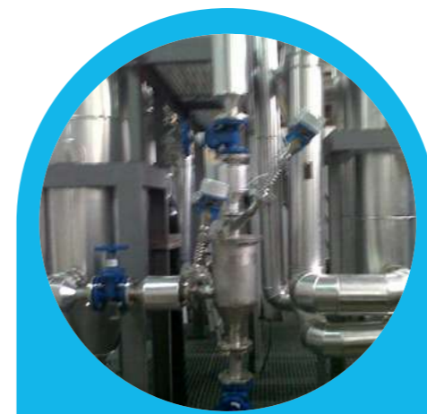
Particle Removal System
