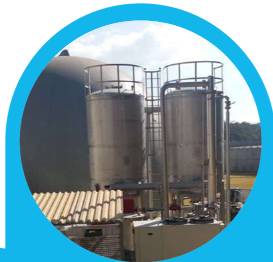
Overview of the plant
