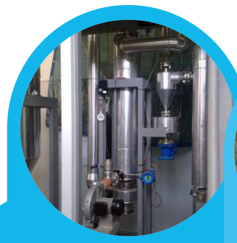
Heat Recovery System
