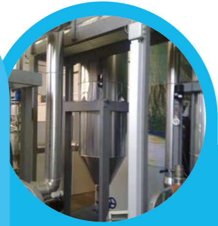
Gas Cleaning System
