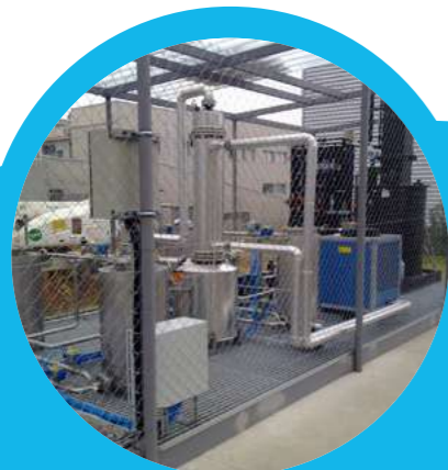
View of energy recovery.
