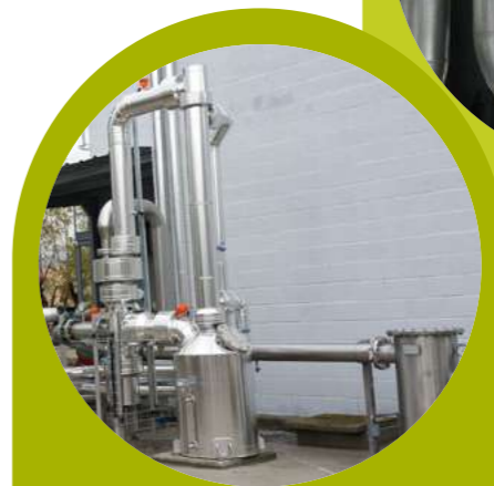
Outside water vapor removal
