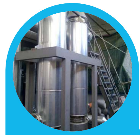
Heat Recovery System
