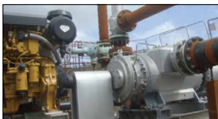
Heavy Crude Oil - Oman Flow - 55 m 3 /hr, Pressure - 16 bar
