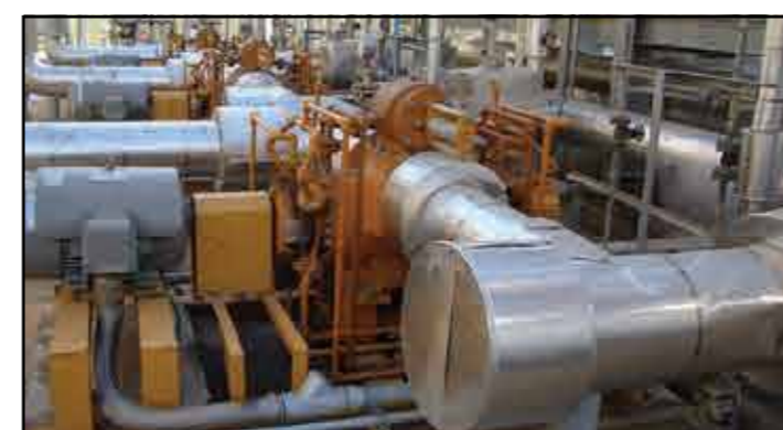
Tar at Steel Plant - South Korea Flow - 110 m 3 /hr, Pressure - 3.6 bar
