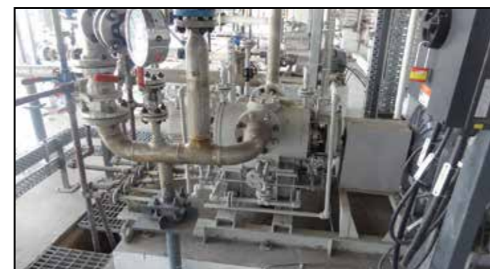
Polystrol Oil at Chemical Plant - India Flow - 30 m 3 /hr, Pressure - 4.5 bar
