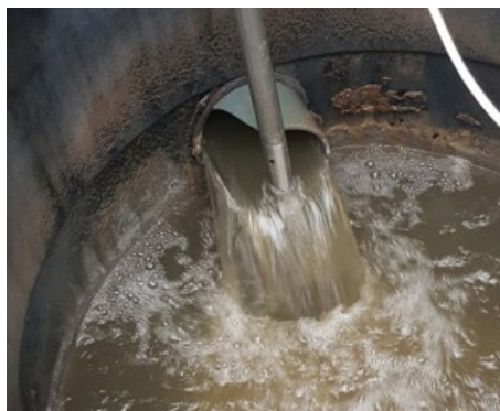
The SulfiLogger™ sensor measured in the liquid sewage at the inlet of the well.
